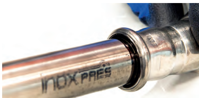
Figure 33 - Example of Incorrect Marking
